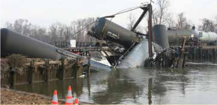
In November 2012 a bridge near Paulsboro, NJ, collapsed sending four DOT-111 tank cars of vinyl chloride into Mantua Creek. Photo: NOAA
